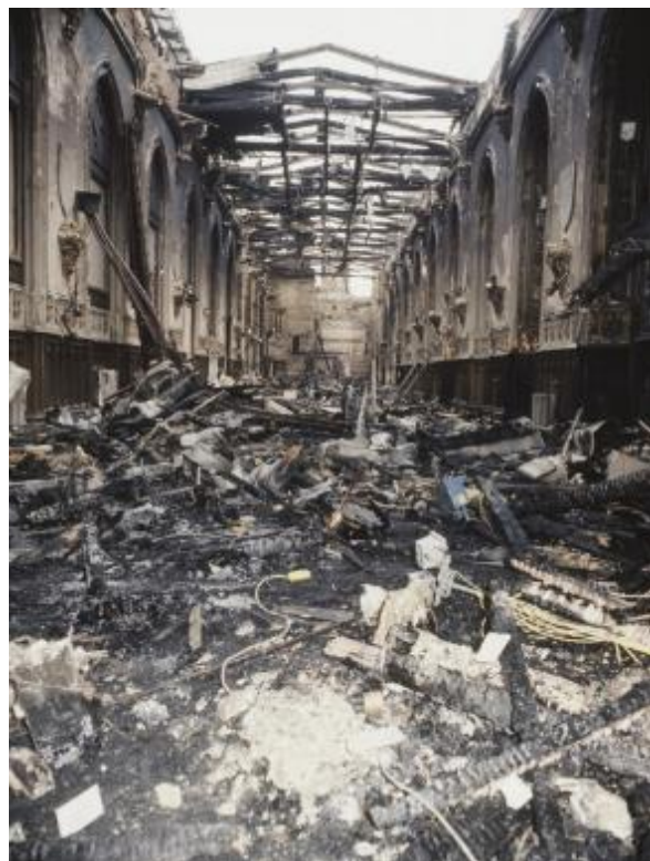
St George's Hall after the fire
