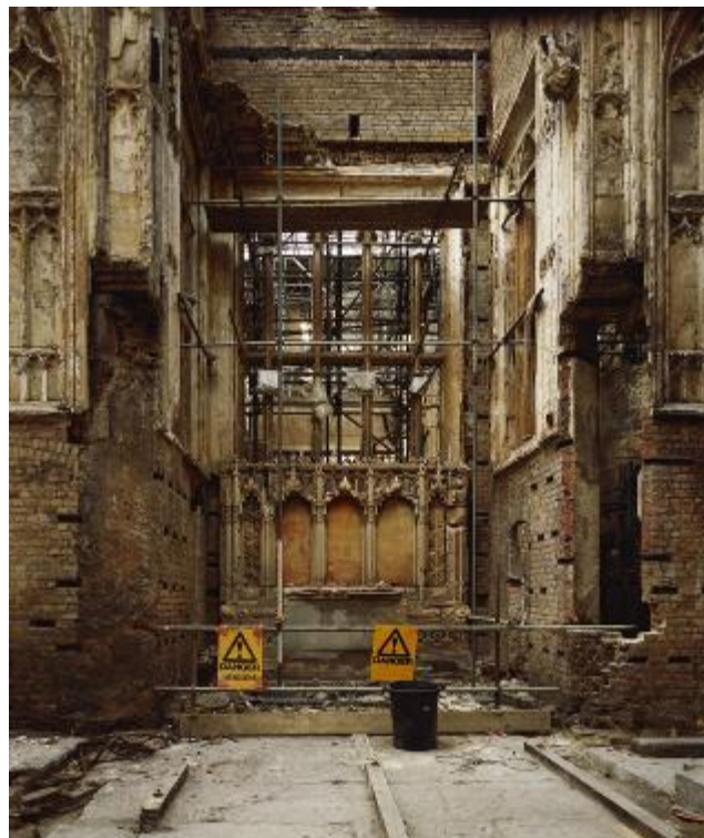
Queen Victoria's Private Chapel after the fire
