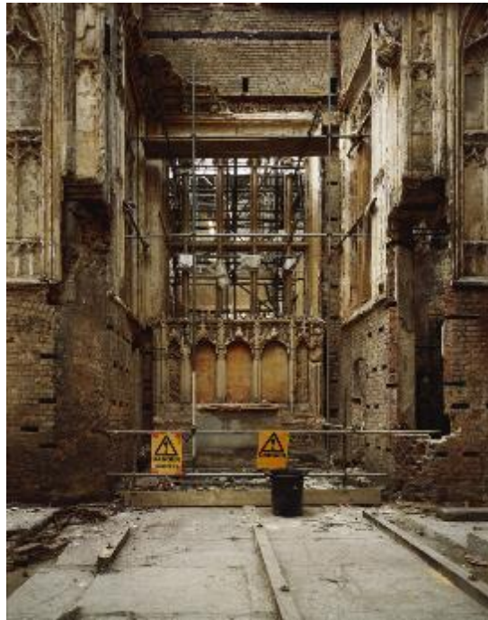
The Private Chapel after the fire
